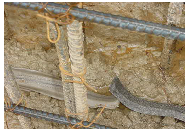
BAD INSTALLATION AND DETAILING
