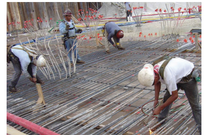
POST INSTALLATION DAMAGE
