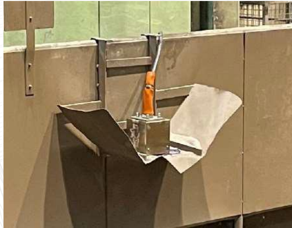
RADAR sensor mounted on a traverse.
