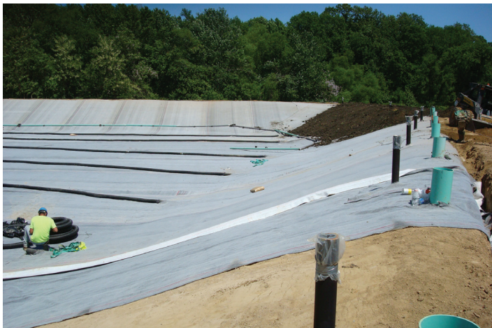
Figure 3-1. Installation of BENTOMAT CL in a typical wastewater lagoon. Inlet pipes in foreground.
